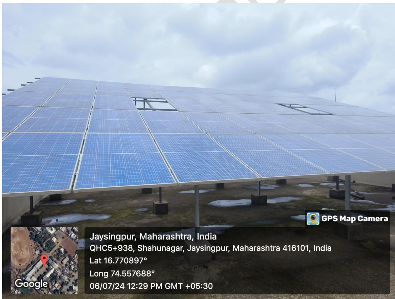
Plate 5: Rooftop solar panels in the premises
