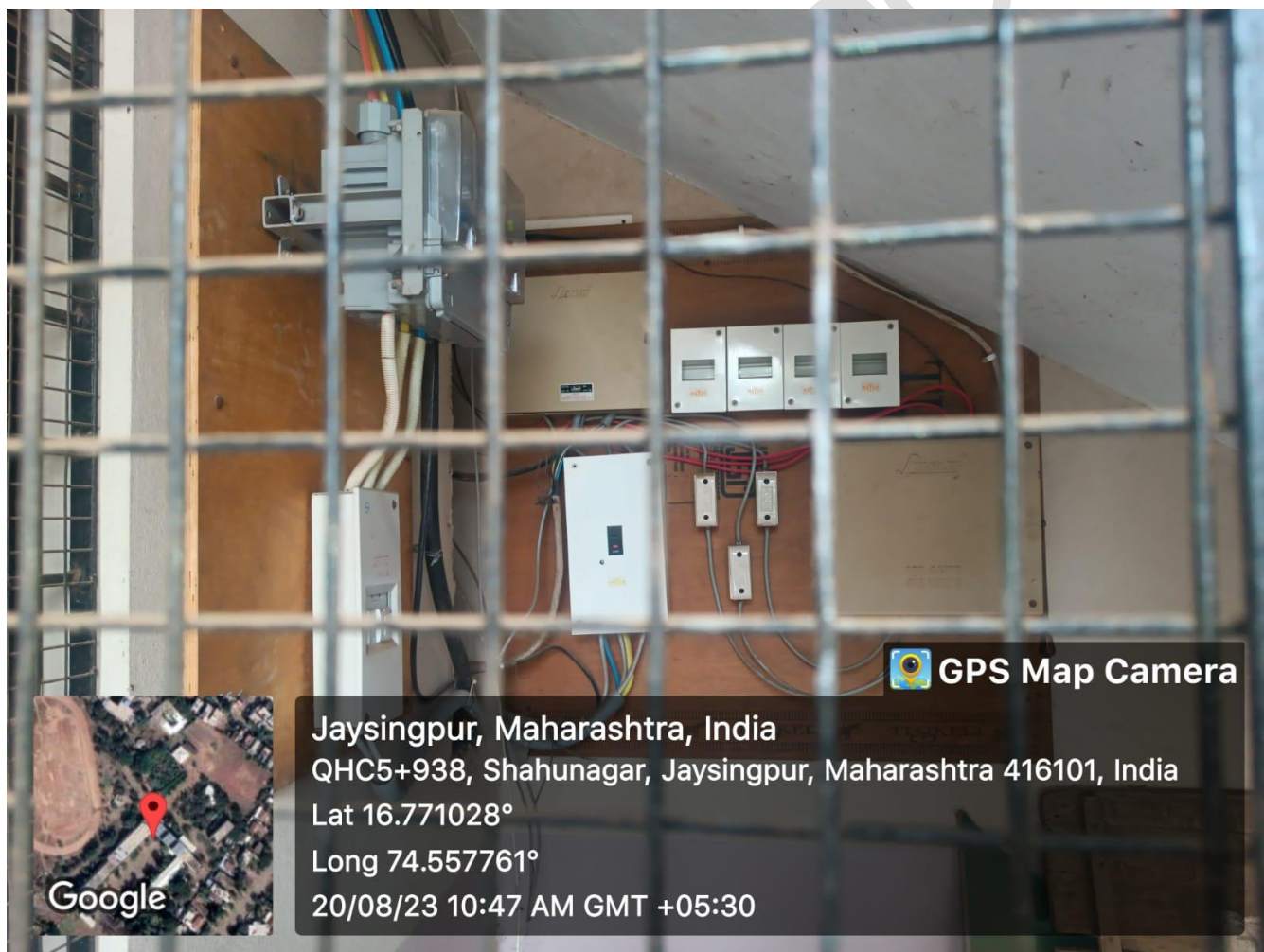
Plate 7: Electric metering system in the premises
