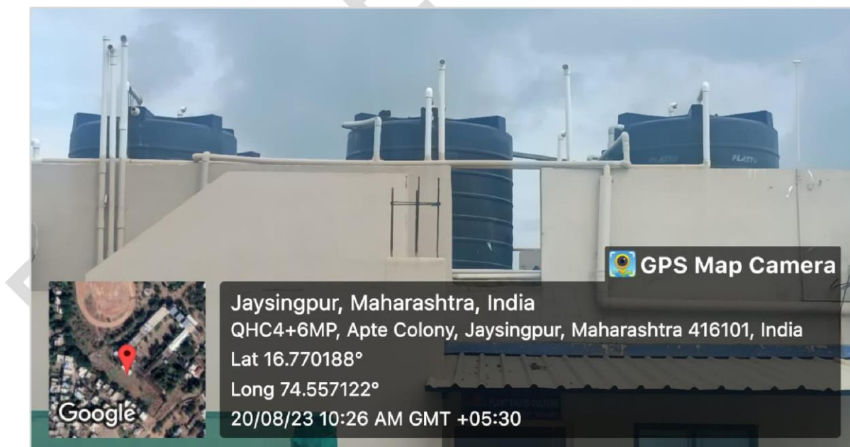
Plate 8: Water facility in the premises
